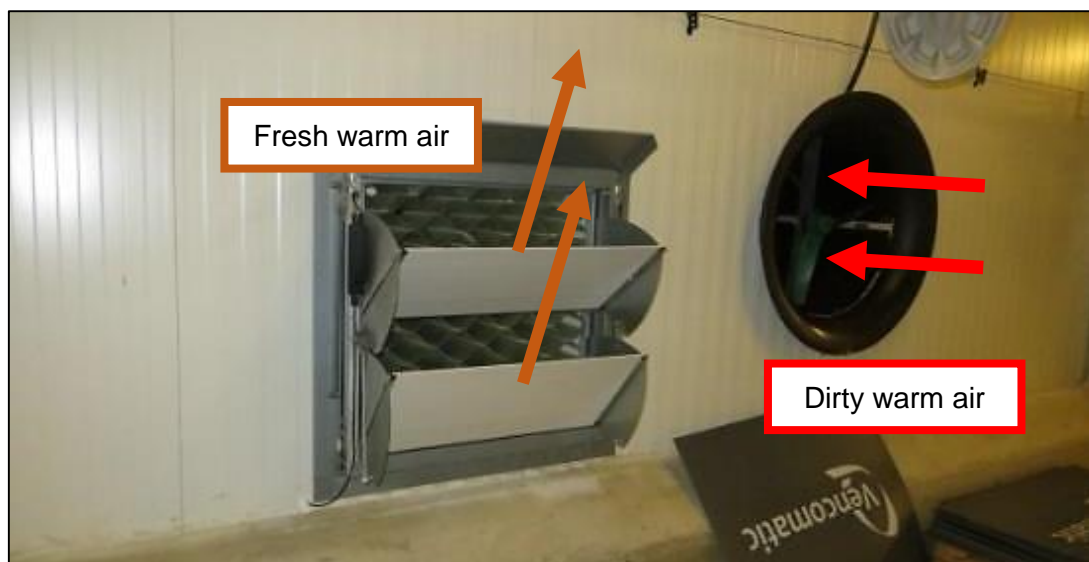
Fig. 43: Heat exchanger - view from inside of the building, Source: Own illustration
