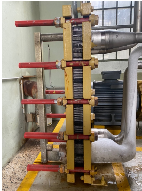
fig. 9: Plate heat exchanger from the CO 2 liquefier; source: own representation.
